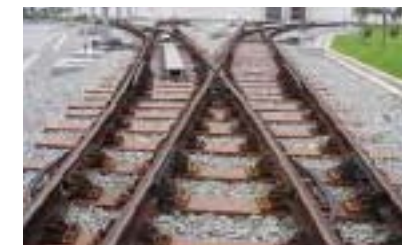
FFU railroad ties at the rail yard for the Guangzhou subway No.8 line
